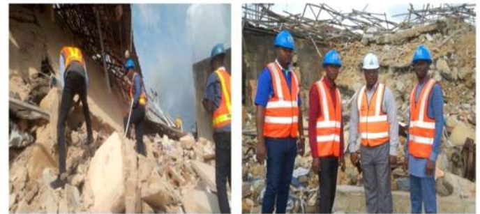
Figure 3: NBRI and Building Collapse in Nigeria (i) 1-Storey at Bukuru and (ii) Imam Street, Uyo
